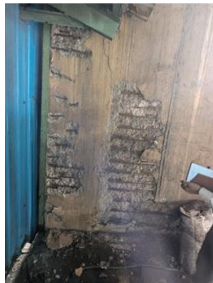
Delamination, spalling of cover concrete and rebar exposure
