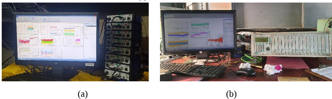
Fig. 3: High accuracy data acquisition system of (a) Bridge No.78 and (b) Bridge No.95
