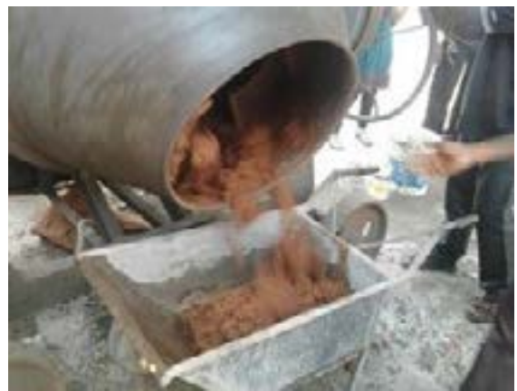
Typical mixing view
